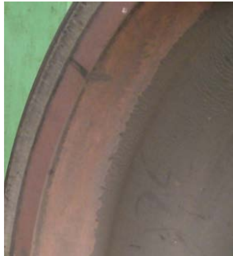
Old and fresh burnt paint
